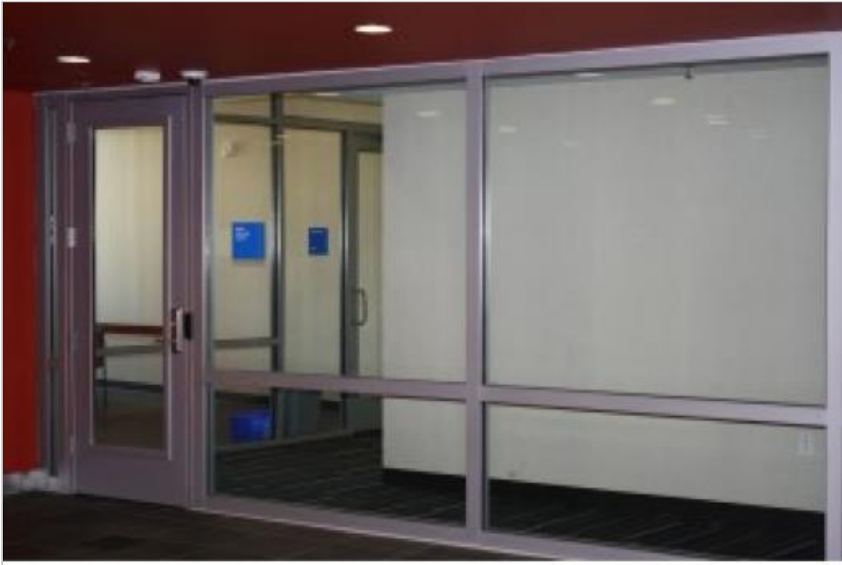
The glazing used in this 1-hour exit corridor exceeds 25% of the wall area. So, 60-minute fire resistive glazing and framing tested to ASTM E-119 was used in the assembly adjacent to the door.
