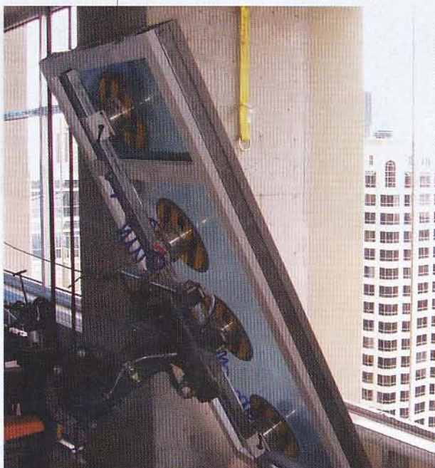
Installation of National Fenestration Rating Council-certified, 45-minute fire-rated window assemblies for Sapphire Towers in San Diego.
